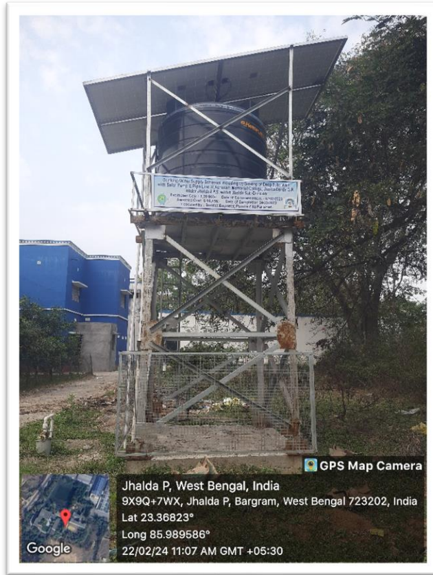
Solar Pump fitted Underground Boring with Water Tank
