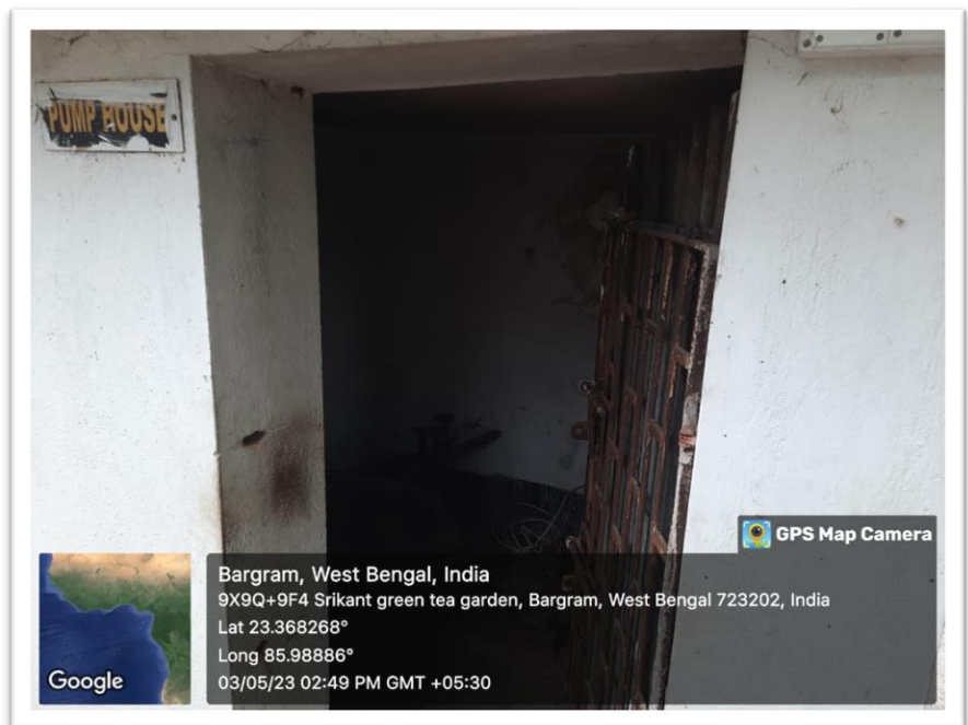
Pump House of Bore Well
