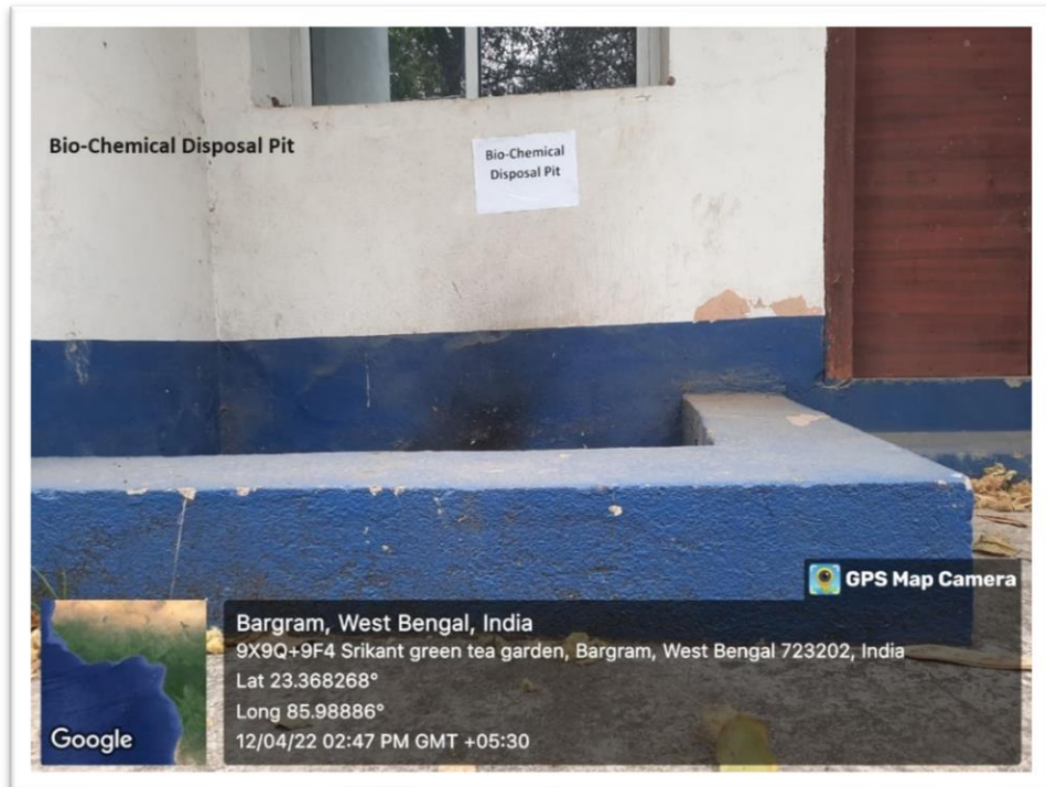
Bio-Chemical Disposal Pit
