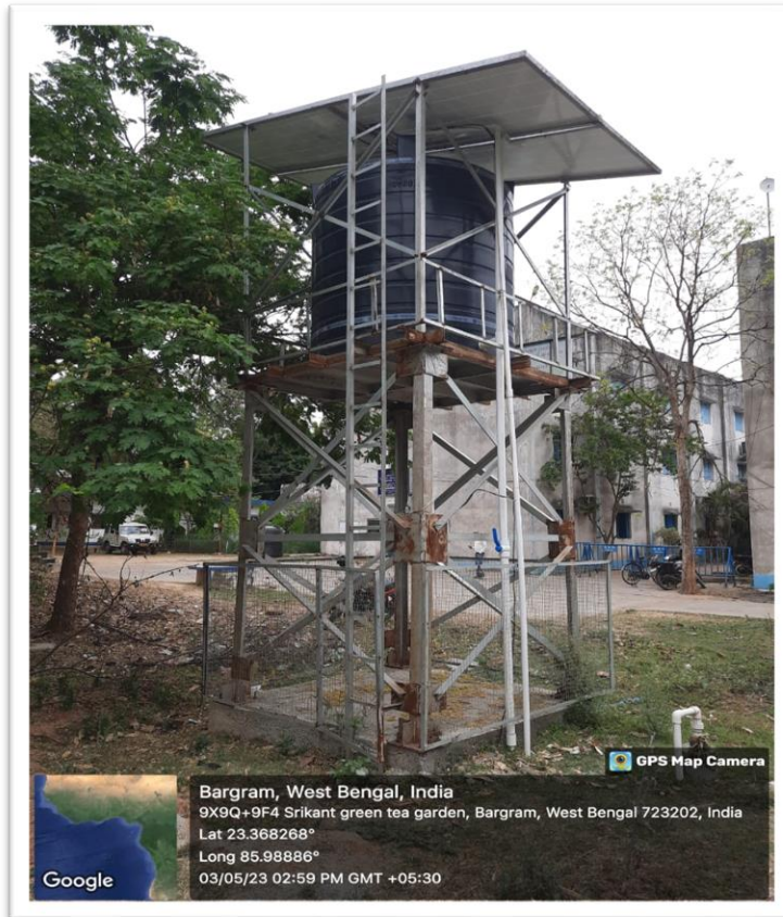
Solar Pump fitted Underground Boring with Water Tank
