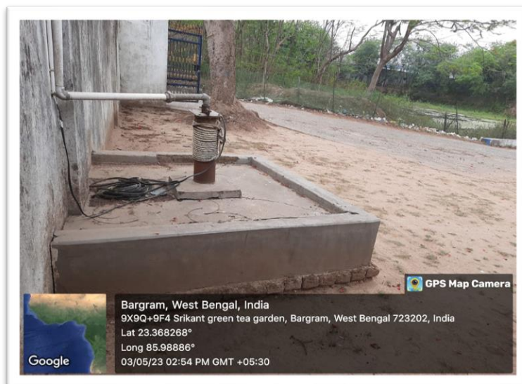
Electric Pump fitted Deep/Underground Boring
